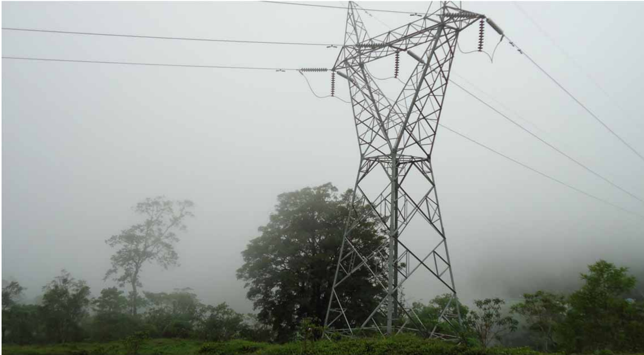
OLP – Transmission Line (Right-of-way) National Grid Corporation of the Philippines (NGCP)
