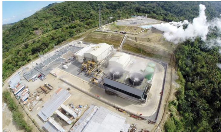
20-MW GEOTHERMAL POWER PLANT (MAIBARARA GEOTHERMAL, INC. - JOINT VENTURE WITH PETROGREEN AND PNOC-RC)
