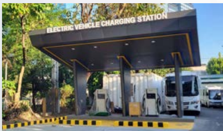
Figure 45. EVCS at the Department of Energy, BGC, Taguig City
