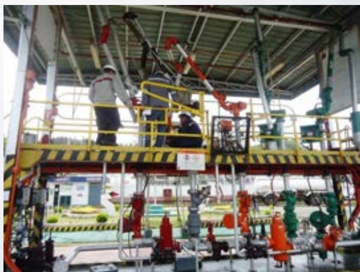
Figure 36. Tank truck loading rack in a liquid petroleum depot
